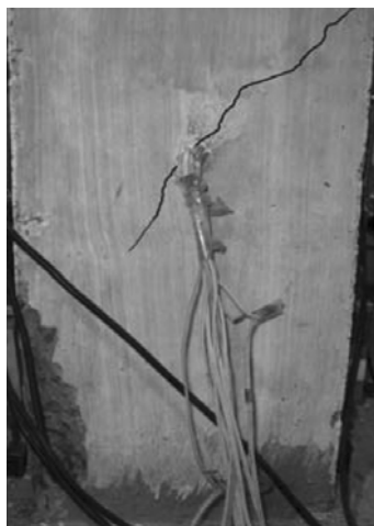
(a) formation of diagonal crack
