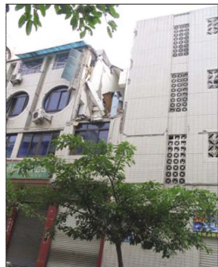
Fig. 19 Partial collapse of building due to knocking along the partition (VII/VIII)
