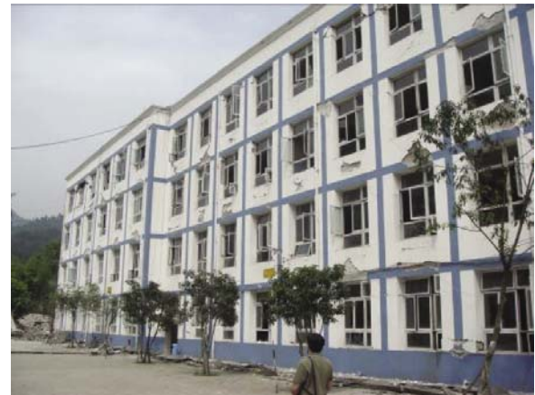
Fig. 13 Damaged masonry school building in Bailu (VII/VIII)
