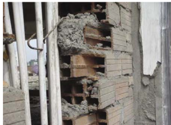
Fig. 23 Damaged infilled wall of perforated brick of a school building in Dujiangyan (VII/(VIII-IX))
