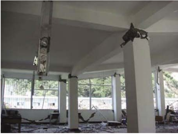
Fig. 7 Plastic hinges at column tops of a dining hall at the ground floor of the Xuankou Middle School in Yingxiu Town (VII/XI)
