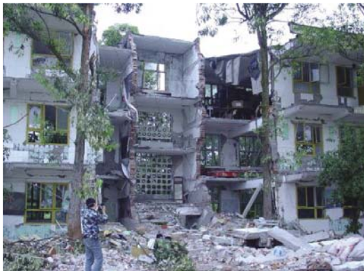
Fig. 15 Collapsed stair shaft of a three-story school building in Mianzhu County (VII/(VIII-IX))
