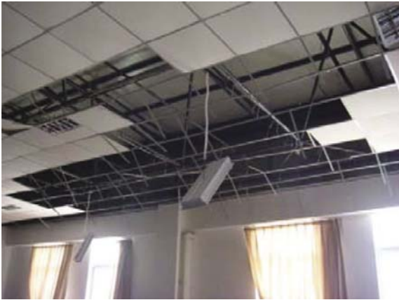
Fig. 24 Damaged ceiling of a school building in Deyang City (VI/VII)
