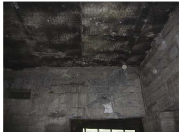
Fig. 10 Damaged high coupling beam of a shear wall structure in Pengzhou City (VII/VII)
