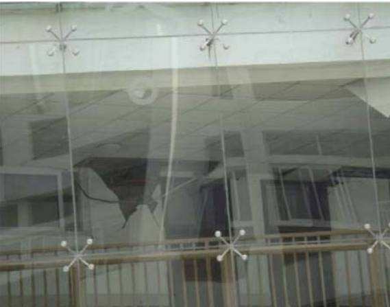
Fig. 25 Glass cladding of a school building remains intact in Dujiangyan (VII/(VIII-IX))
