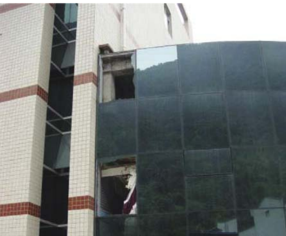
Fig. 26 Two slices of glass fell down from the cladding in Anxian County (VII/IX)
