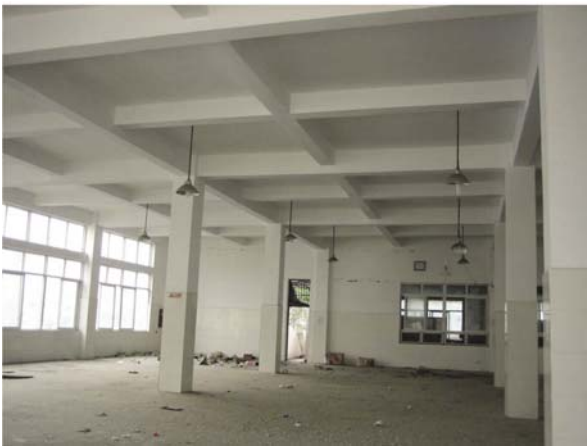
Fig. 8 The dining hall at the second floor of the building shown in Fig. 7 remains intact
