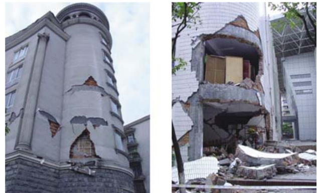
Fig. 22 Failure of walls at the corner of two buildings (VII/VIII)
