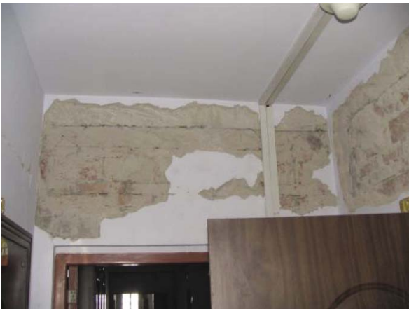
Fig. 12 Twin coupling beam of a frame-shear wall structure in Xi'an City (VII/(VI-VII))
