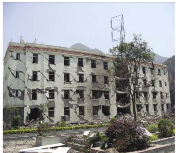
Fig. 3 Damaged official building in Yingxiu Town (VII/XI)
