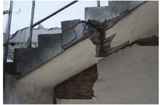
Fig. 17 Fractured stair beam at its lower 1/3 position (VII/(VIII-IX))
