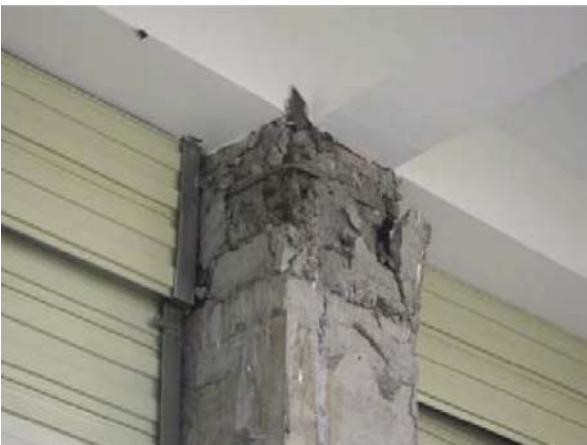
Fig. 9 Plastic hinge at the top of a column (VII/XI)
