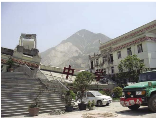
Fig. 1 Collapsed school building (left) in Yingxiu Town (VII/XI) (Note: VII/XI means the specified intensity /estimated intensity and same below)
