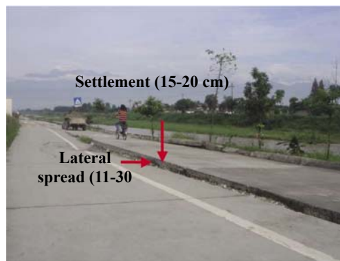
(d) Settlement and lateral spreading of road (P4)
