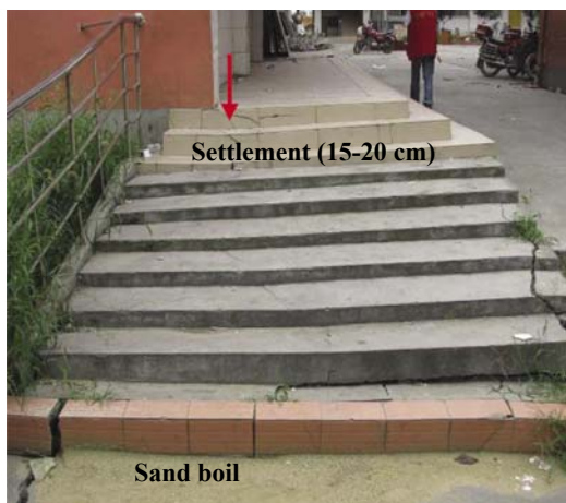
(a) Settlement of the east corner (P1)
