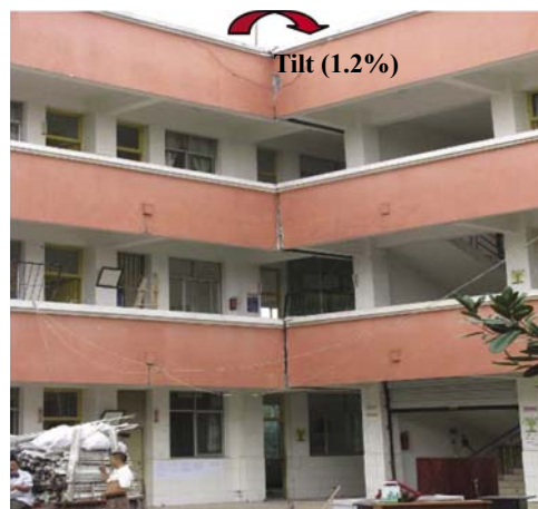
(b) Tilt and knocking of two adjacent buildings (P2)
